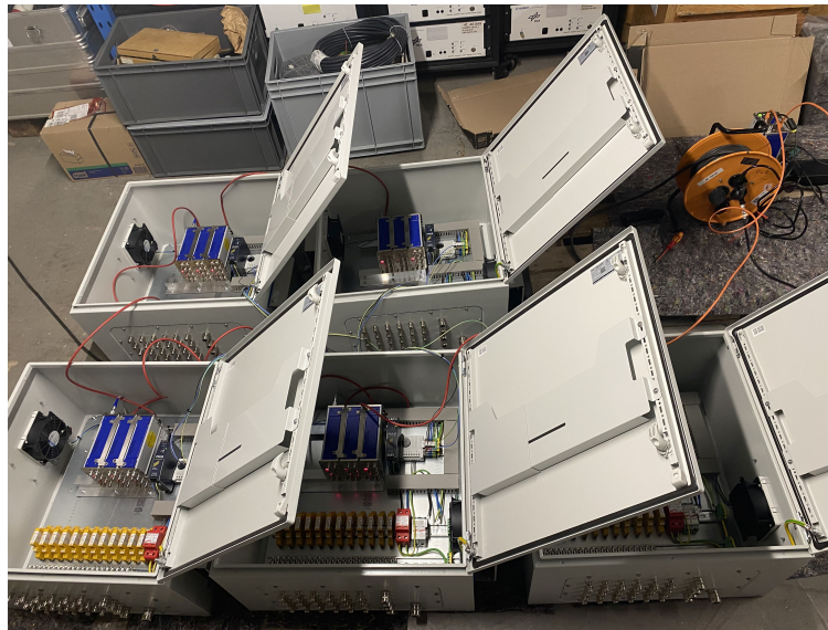
Figure 4: Final check of control cabinets before the installation. The measuring modules are connected to each other with a patch cable.
