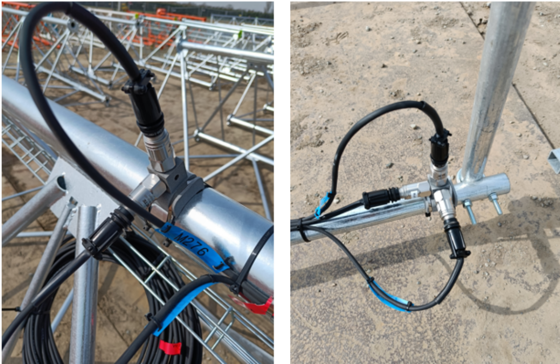
Figure 2: Instrumentation of the sensors on the ground at the construction site. Left: biaxial measurement point on a mast segment. Right: triaxial measurement point at the end of a boom tube.
